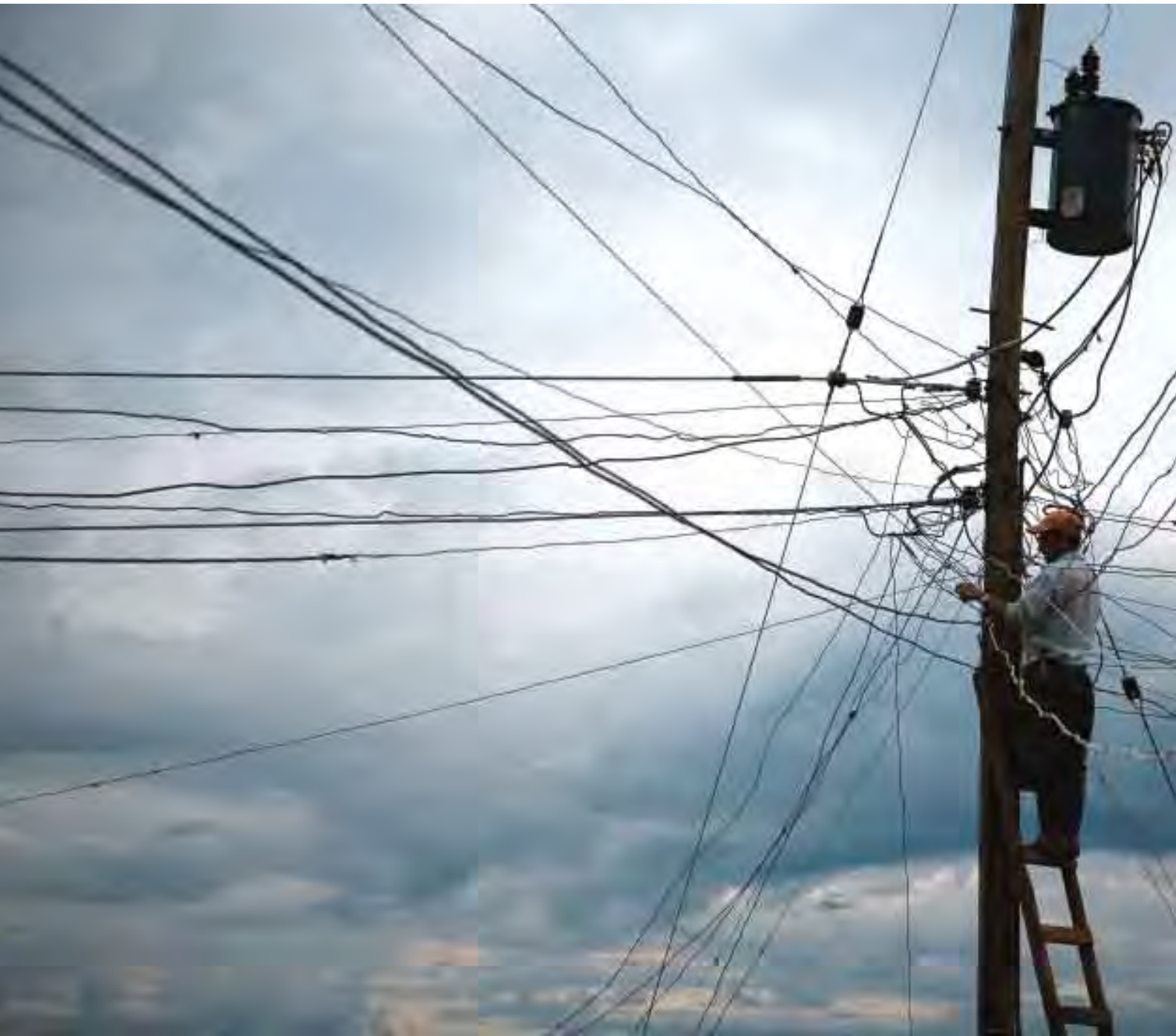
A man draws an electrical line to his home from the only power line running through El Pacifico, an informal settlement on the outskirts of Medellín, Colombia.
